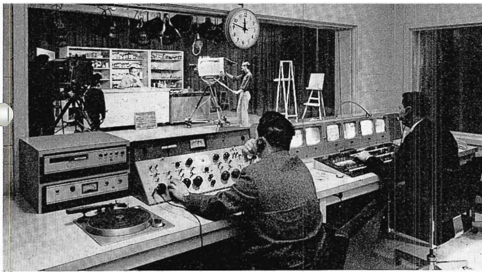
PRODUCTION CONTROL CENTER designed by station technical staff using RCA "New Look" equipment. Personnel monitor audio and video; perform switching to record programs on television tape. Equipment (L to R) consists of RT-7 Cartridge Tape (and turntable), BC-8 Audio Console, TS-40 Program Switcher.
